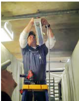
Electricians, Brad Eveland and Doug Dahl, prepare conduit to install an LED light fixture in the Artifact Preservation Center. Sixty-three florescent fixtures were upgraded to LED during this process.
