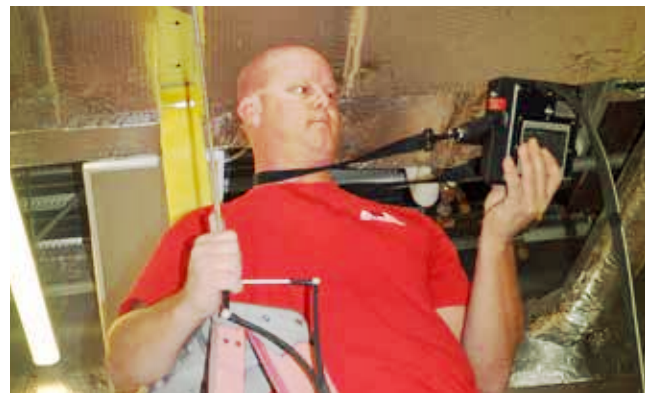
Re-commissioning crew member, Corey Evans, measures air flow through a major duct line to confirm the return fan is properly working. Air ducts for all four of the museum’s air handling units were evaluated, and fan adjustments were made as needed.
