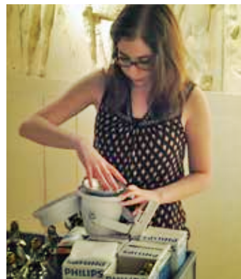
Student employee, Scarlett Andes, installs LED bulbs in light fixtures to be installed in gallery track lights. A total of 1,140 gallery lights were upgraded during this process, both inside cases and in room-ambient light fixtures.
